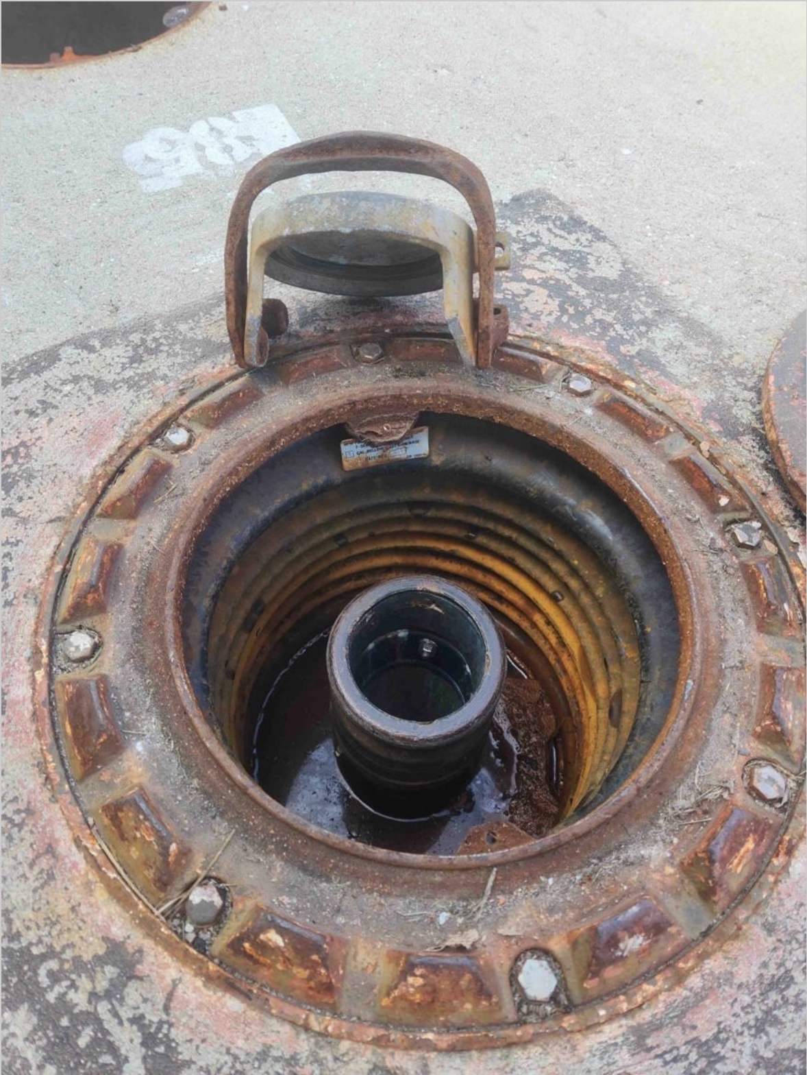
Spill bucket components
